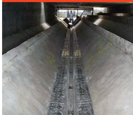
Fig. A.4.5-2 Waste water heat exchanger
